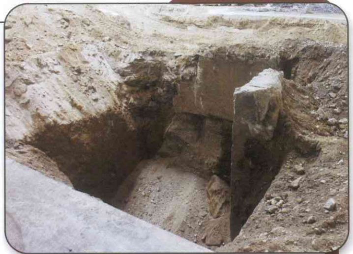
Abandoned reinforcing walls at Cal Steel's Fontana plant for what had once been the underground power rooms for Kaiser Steel's 1940s-era galvanizing operation.
