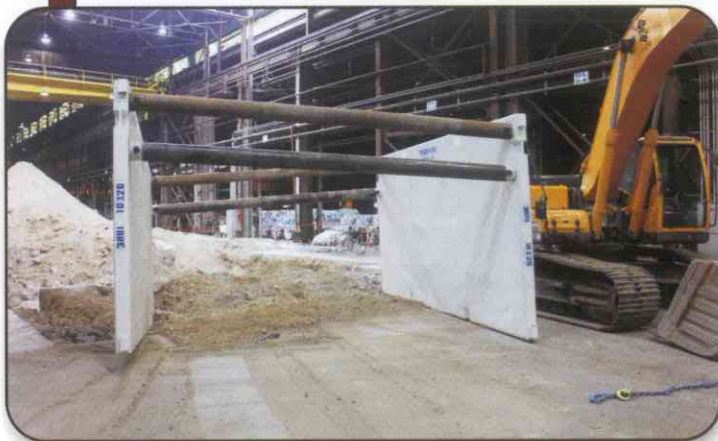
TPR delivered trench boxes, beams and 8' X 20' steel plates to the job for the 20' deep excavation.
